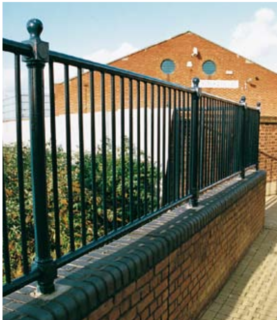
▲ REIGATE FULL GUARDRAIL
